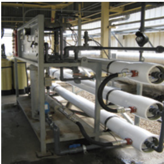
3. Reverse osmosis improvements reduce consumption of city water, electric bill (access presentation 10)
