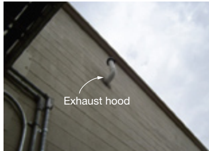
35. Weather hood guards ventilation system against the elements
