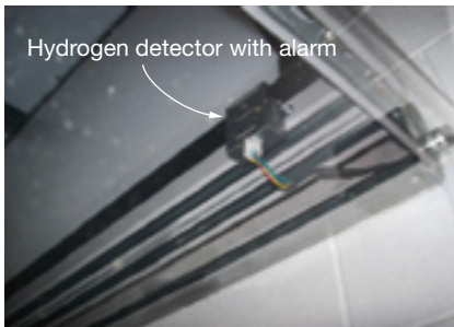
34. Safety is assured by hydrogen detector equipped with an alarm
