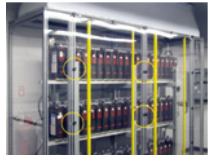
32. Flooded-cell battery system has Teflon® hood for electrical insulation, ventilation holes at the base to ensure air flow across the batteries, and special hinges (circles) to facilitate removal of doors for maintenance
