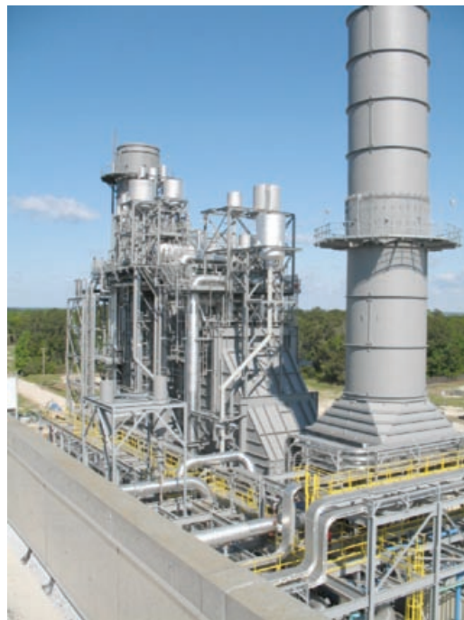
1. Downstream of the gas turbine is the bypass stack and the heat-recovery steam generator for the repowered Hopkins Unit 2
